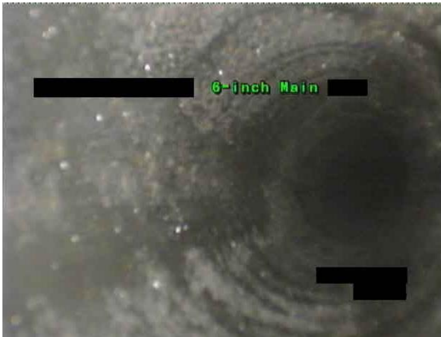
Figure 2. Video-borescope screen capture showing no corrosion other than normal zinc oxidation in pre-action system without residual water.
